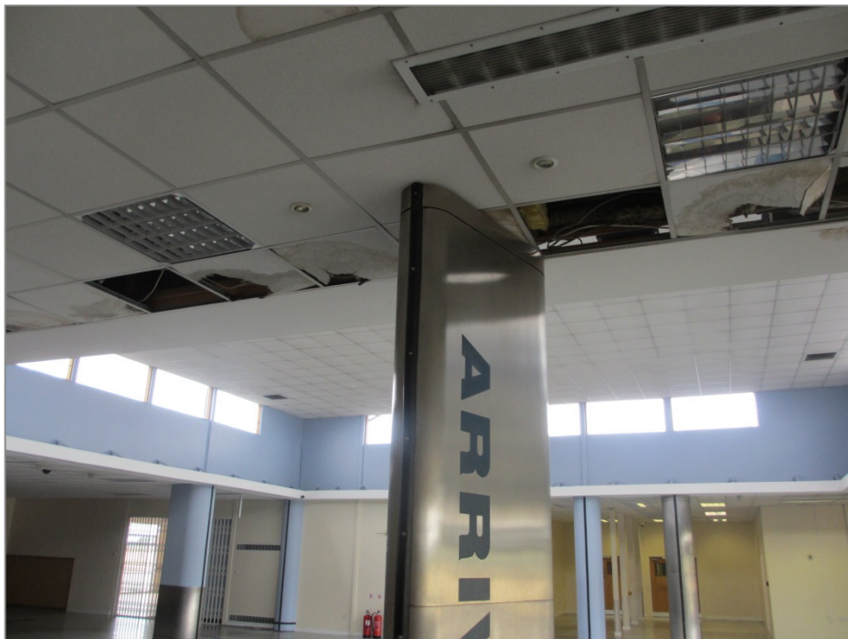
Figure 4: Evidence of water damage in may foyer.
