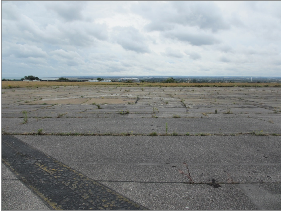
Figure 10: Shoulders of runway are paved. Evidence of plants establishing a presence in cracks
